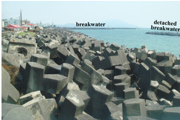
Fig. 10. Coastal prevention work using a stockpile of armored blocks causing water depth to be deeper in front of revetments at Kezailiao Coast.
