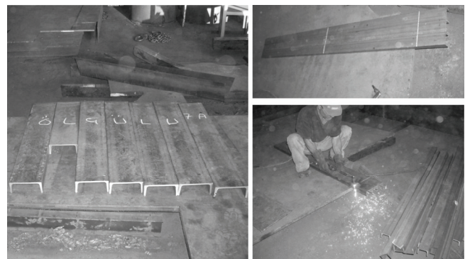
Fig. 2. The marking of the cutting patterns and cutting of U-section channel beams.
