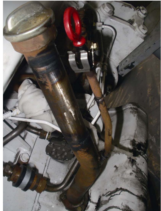
Fig. 11. Oil dipstick pipe, its clips and oil mess.
