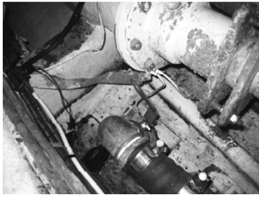
Fig. 24. Pipes and electrical continuity of these links horn cap and bottom valves.
