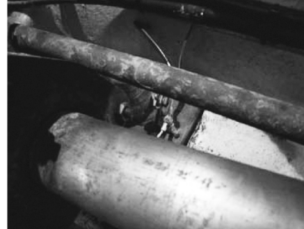
Fig. 10. Untreated copper pipe.
