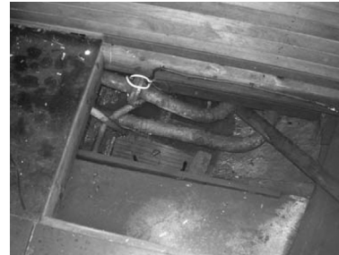
Fig. 22. Pipe corrosion in services.
