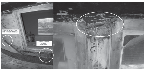
Fig. 25. Corrosion of screws and steel frames in the underwater sight glass windows.
