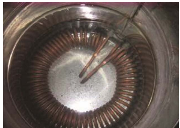
Fig. 13. The heat pump water heater.
