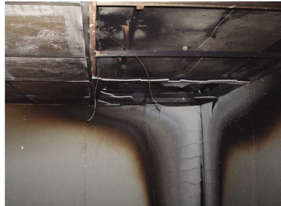
Fig. 5. Penetration of gypsum board beneath the ceiling by the flame from the burner.
