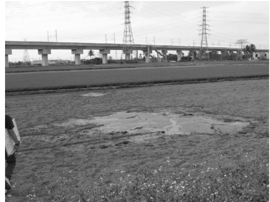
Fig. 4. Silty sand liquefaction at Hsin Hwa site during 2010 Jia Sian Earthquake, Tainan, Taiwan.
