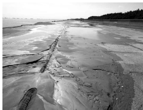
Fig. 3. Silty sand liquefaction at the seaside zone in the south of the Cemetery Park, Urayasu, Japan.
