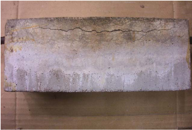
Fig. 3. The photo of the surface crack induced by the alkali-silica aggregate reaction.
