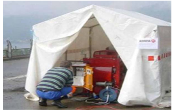
Fig. 6. MMLS3 field testing of bituminous plug expansion joints in a heated tent.
