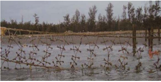
Fig. 8. Short wire fins attached to the wire nets of No. 2 flexible breakwater.
