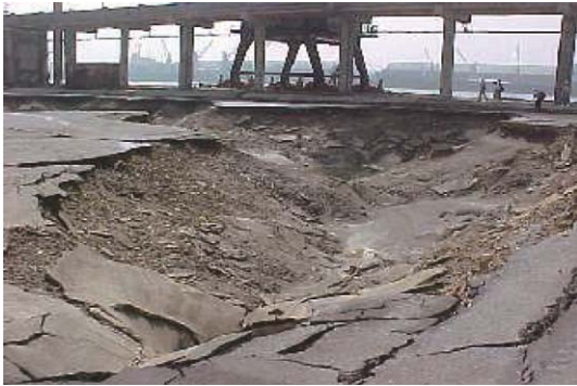
Fig. 2. Large area of liquefaction at a wharf in the Chi-Chi Earthquake, Taiwan.
