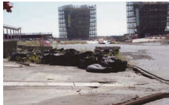
Fig. 1. Large area of liquefaction of a wharf in the Great East Japan Earthquake.
